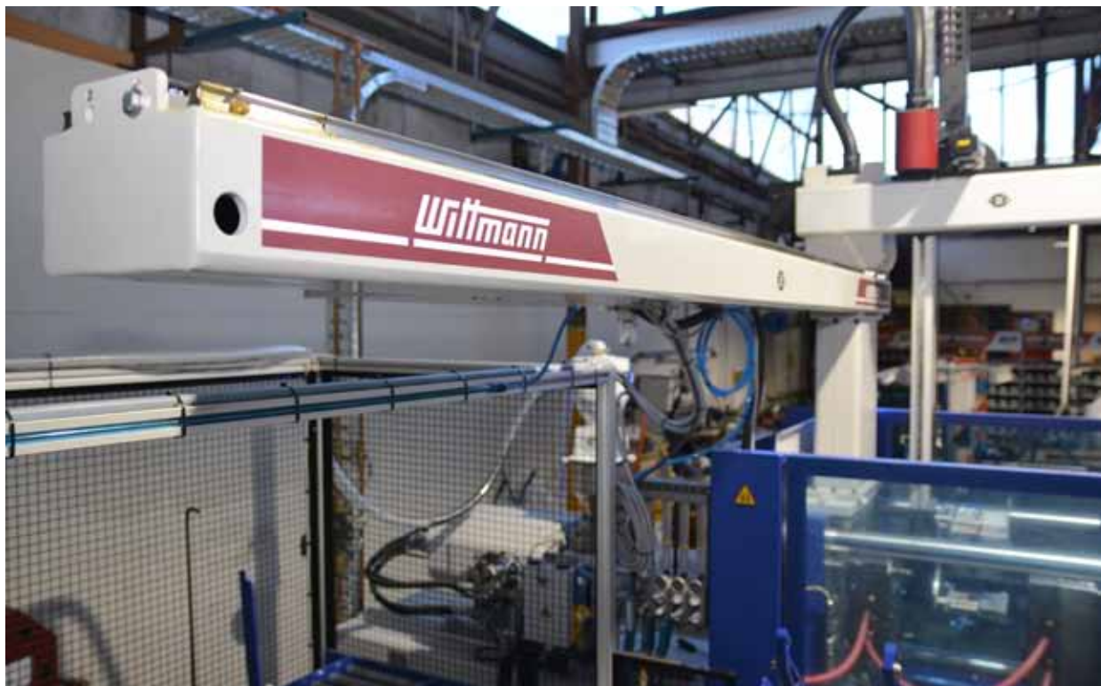
View of an injection molding working cell from the WITTMANN Group, consisting of a WITTMANN BATTENFELD injection molding machine and a WITTMANN robot, installed at MtM Pty Ltd. in Melbourne, Australia.
